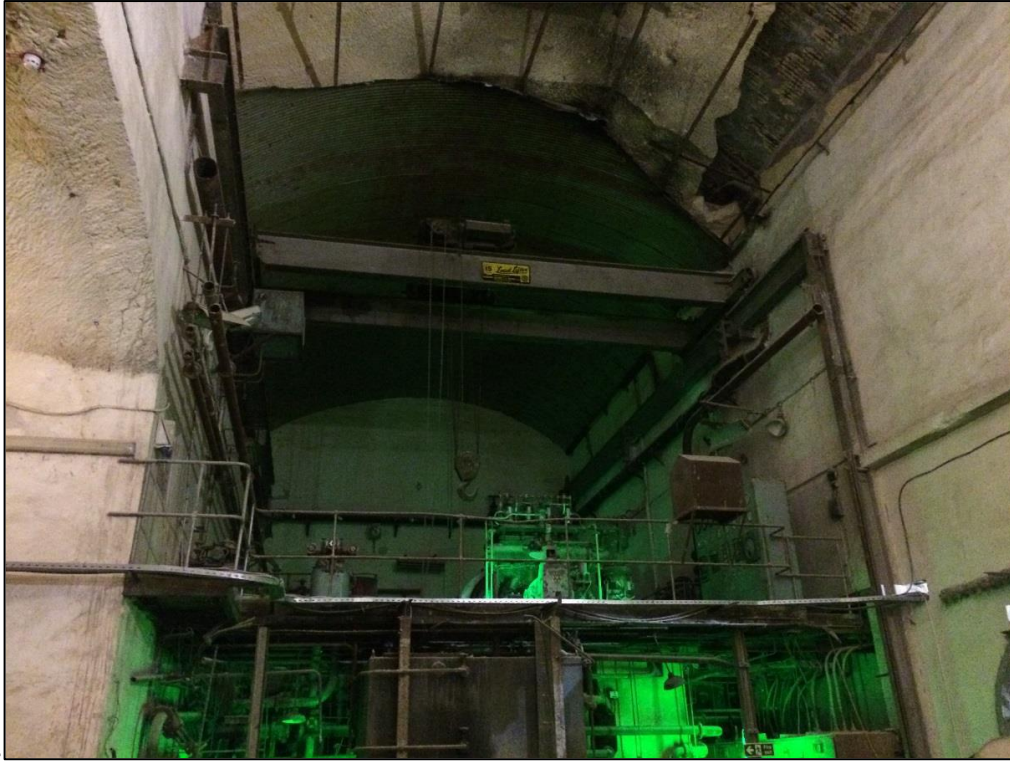
Figure 5: The only remaining turbine located at the far end of the Turbine Hall. This is outside of the area being proposed for the BESS facility (photo dated 2018).
