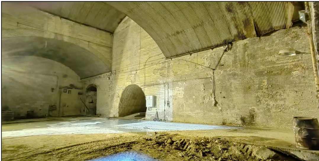
Figure 6: Part of the A-Station tunnel located at the end of the Boiler Hall which is expected to be used for the transportation of the BESS components at the project site. Image also shows the tunnel excavated by PA 3908/08 and PA/05631/16 (photo dated 2023).
